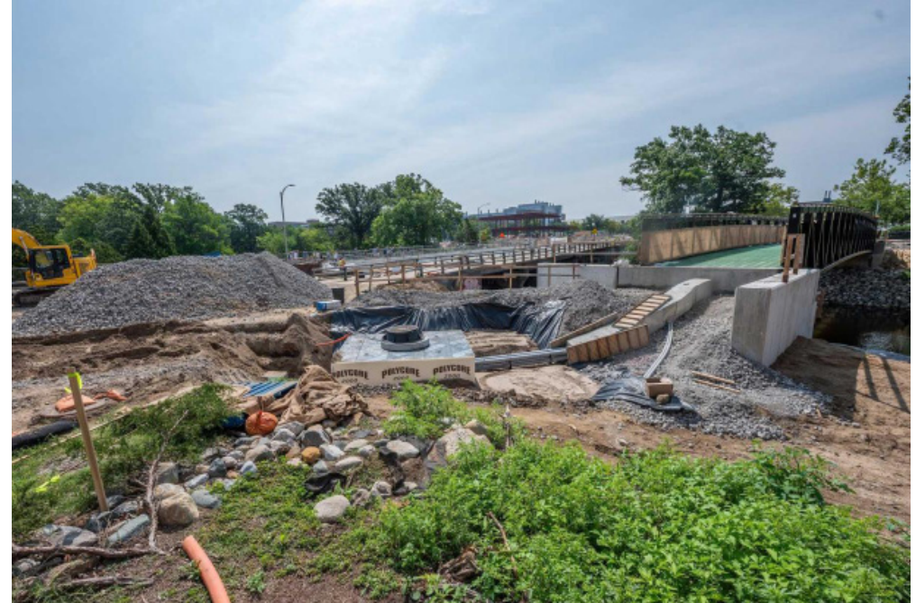
Figure 3-f: Construction of the New Farm Lane Bridge Project, highlighting the new pedestrian bridge to help alleviate foot traffic.
