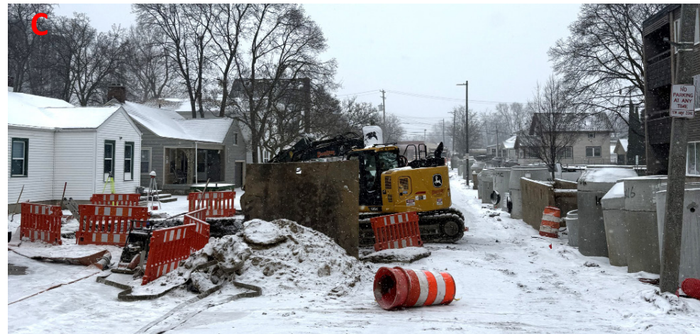
Figure 3-i: Construction staging and utility infrastructure occupying River Street, limiting pedestrian and vehicular movement Phase 1 - Qualitative Analysis
