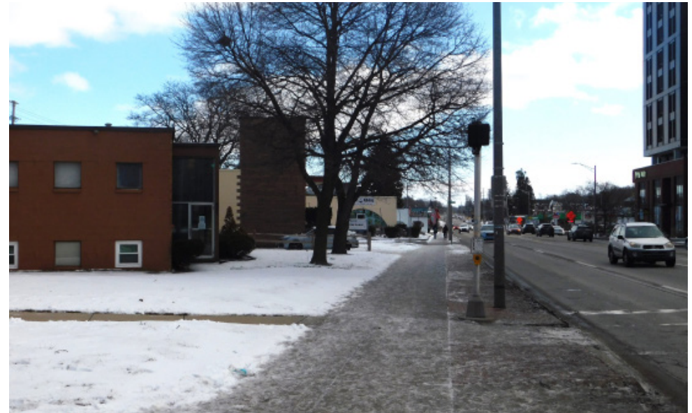
Figure 5-c: Narrow Sidewalk with No Buffer, 1001 E Grand River Ave Photo taken on the NE corner of Grand River and Durand St, facing east
